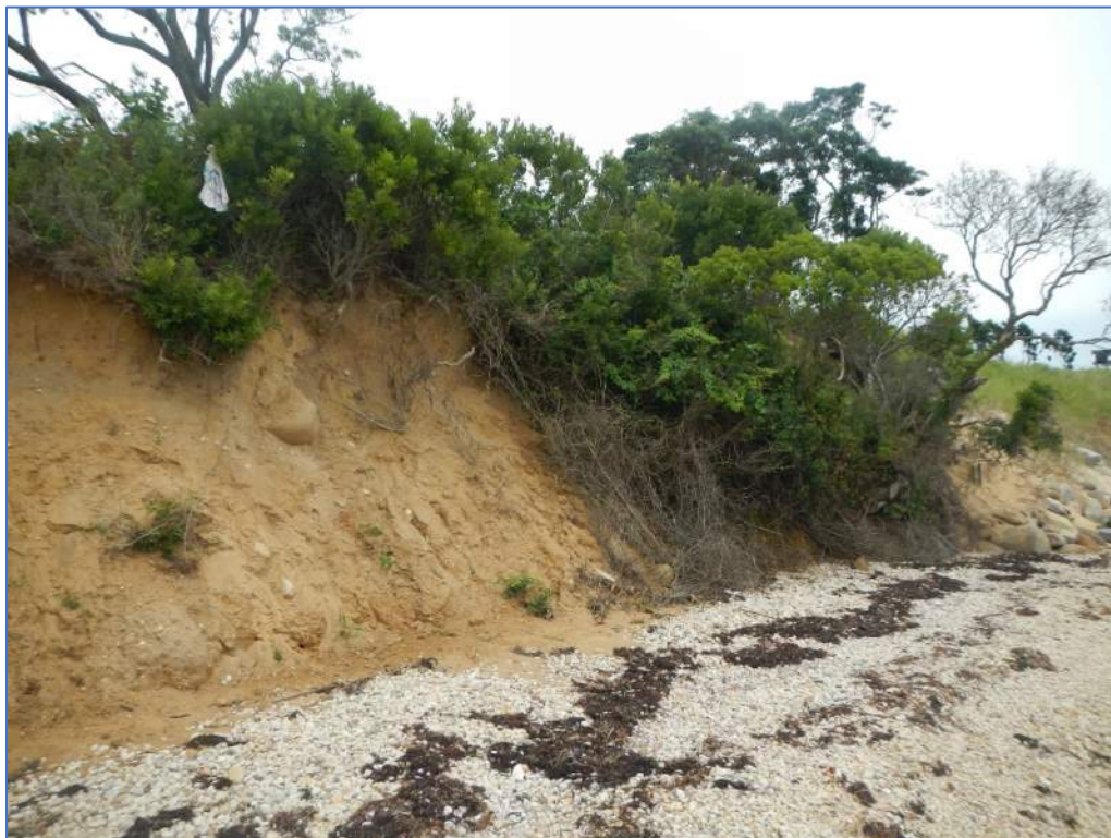
Photograph 26: Eroded – Shoreline Condition (Sheet 3 of 3)
