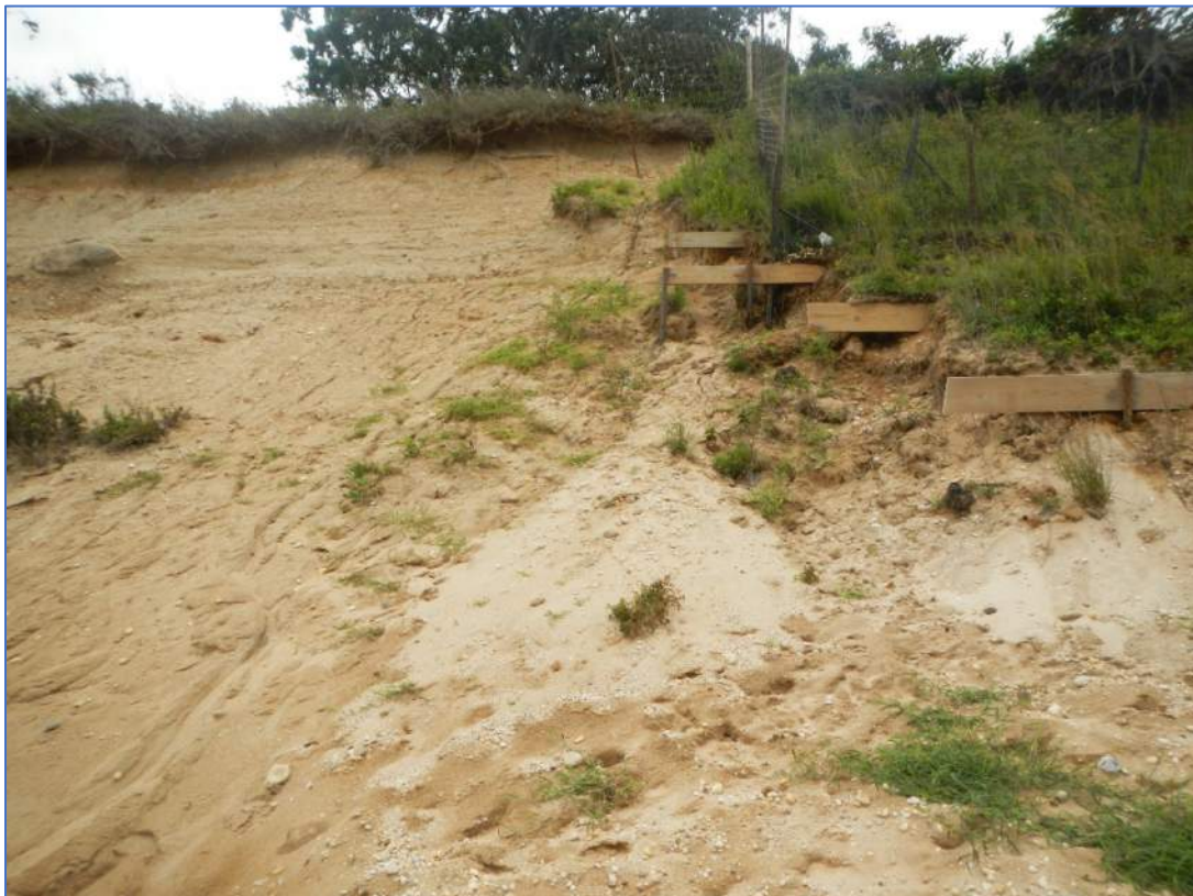
Photograph 28: Critical – Shoreline Condition (Sheet 3 of 3)
